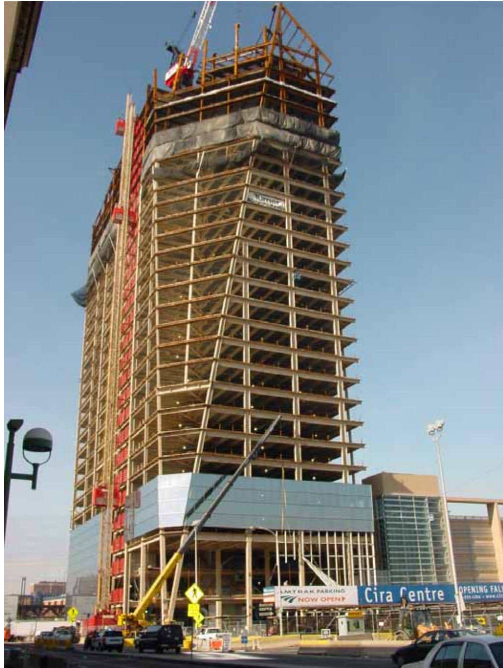
Cira Centre Tower, Philadelphia, PA used Southwest Type 5GP™ and Type 7HD™
