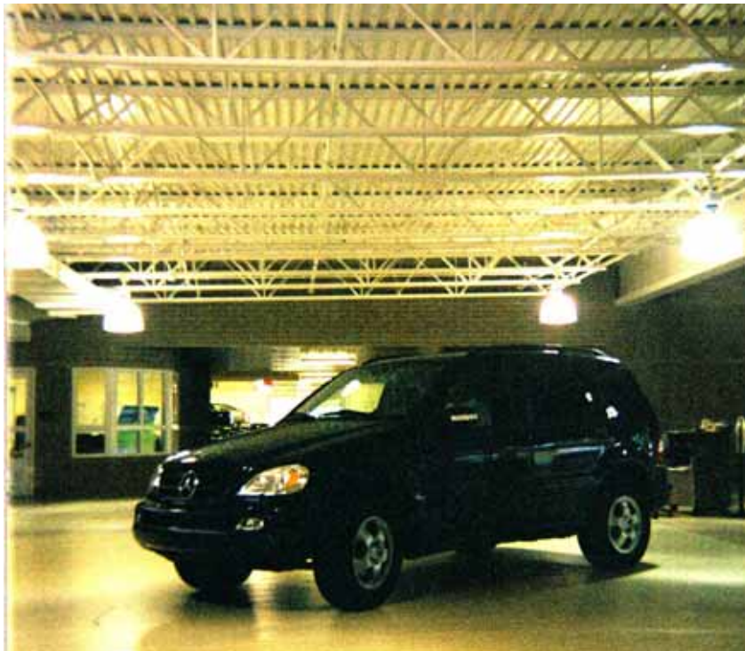
Beams and trusses were coated with Nullifire S606 to achieve the required fire resistance ratings and maintain a stylish “open ceiling” look.
